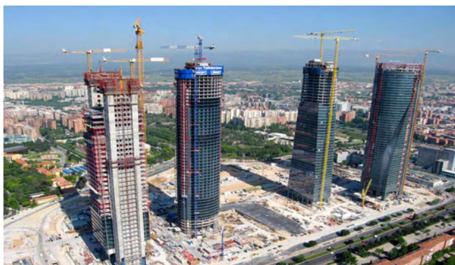
The four skyscrapers at the Real Madrid Sport City (now the "Cuatro Torres Business Area") during their construction.
