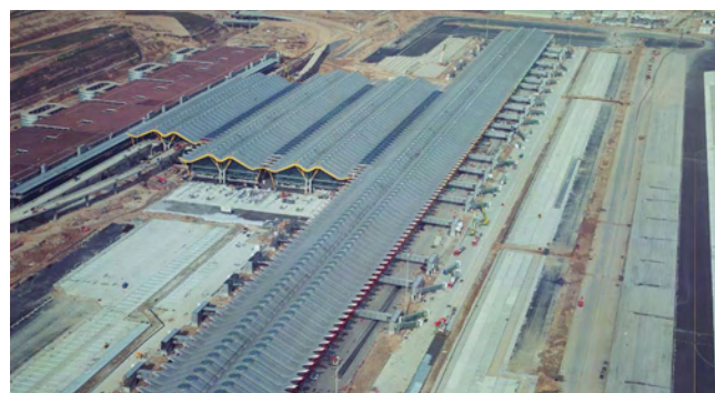
Aerial view of terminal T4 at Madrid-Barajas Airport in its final stage of construction.
